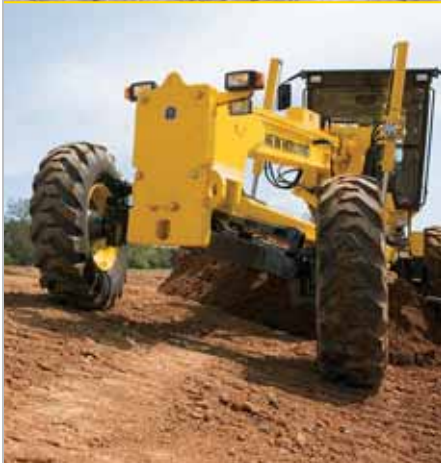
The standard five-position moldboard saddle angle is a natural for grading slopes and embankments.
